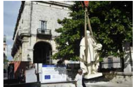
© Office of the Historian of Havana – the statue of King Ferdinand VII is transferred giving room for works in progress
